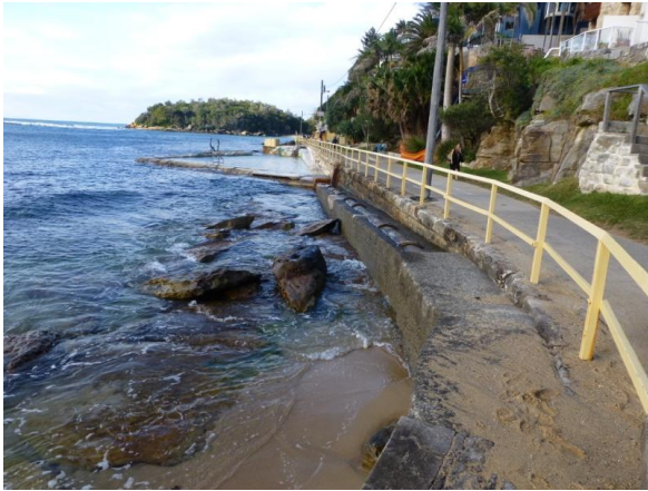
Photo showing exposed stormwater pipe below walkway near Fairy Bower Pool sketch below shows proposed treatment to create public use walkway/seating area
