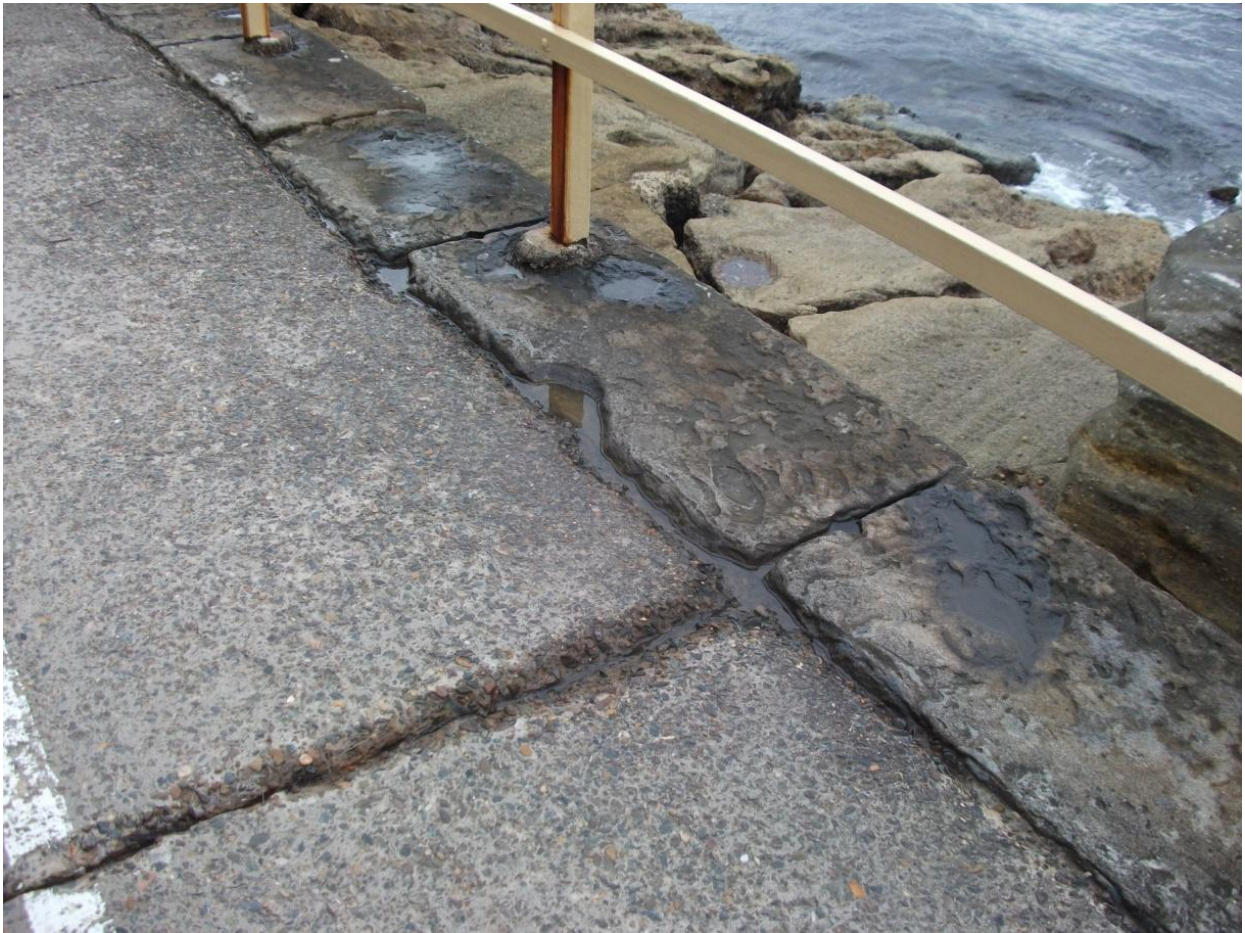
Original concrete pathway slabs now due for replacement
