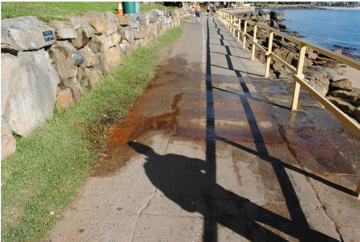
Example of area of concrete pathway suffering from ongoing seepage that now needs to be dealt with effectively and holistically .This ongoing issue would be dealt with as part of the proposed works.
