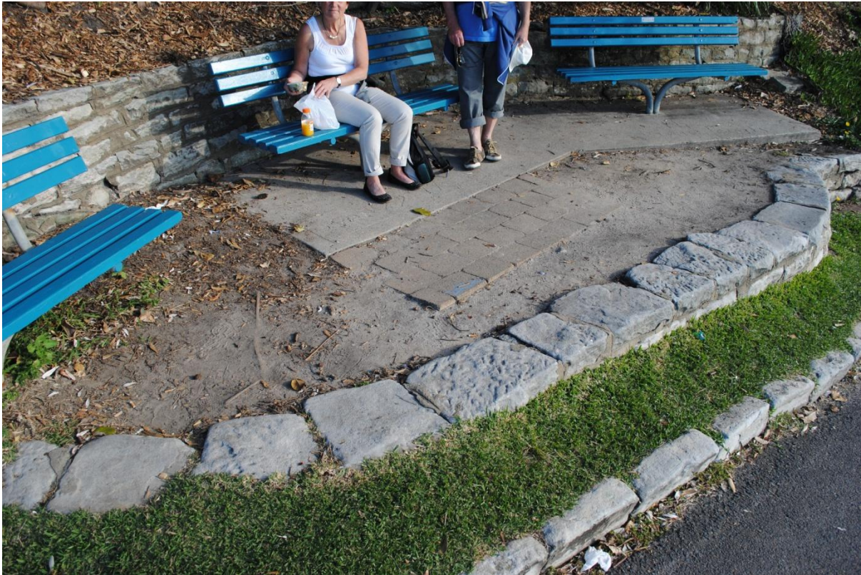
A typical example of deterioration of paved areas associated with public seating spaces. This photo also highlights the need to now replace the outdated furniture type
