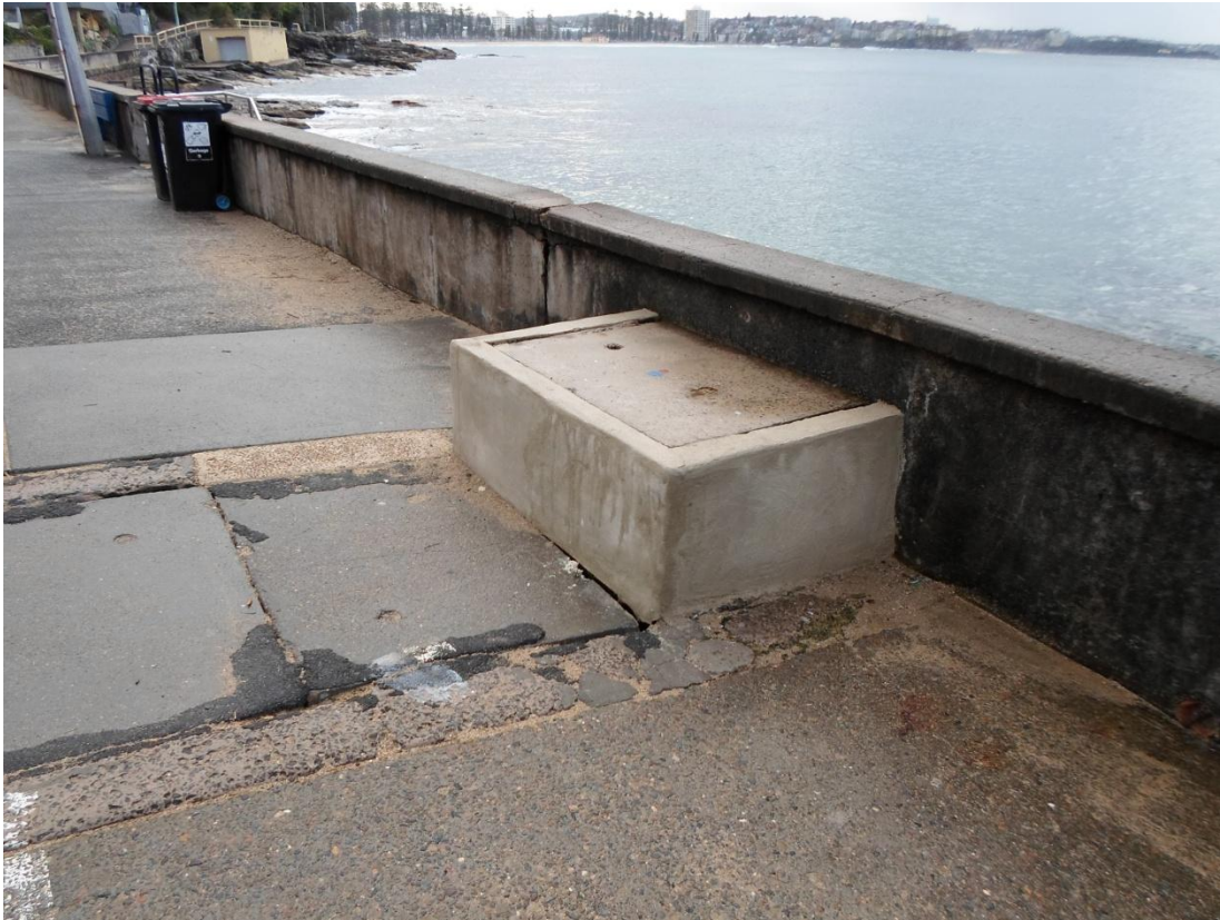
An example of deteriorating storm water infrastructure and unsightly asphalt at the Bower Lane Marine Pde intersection
