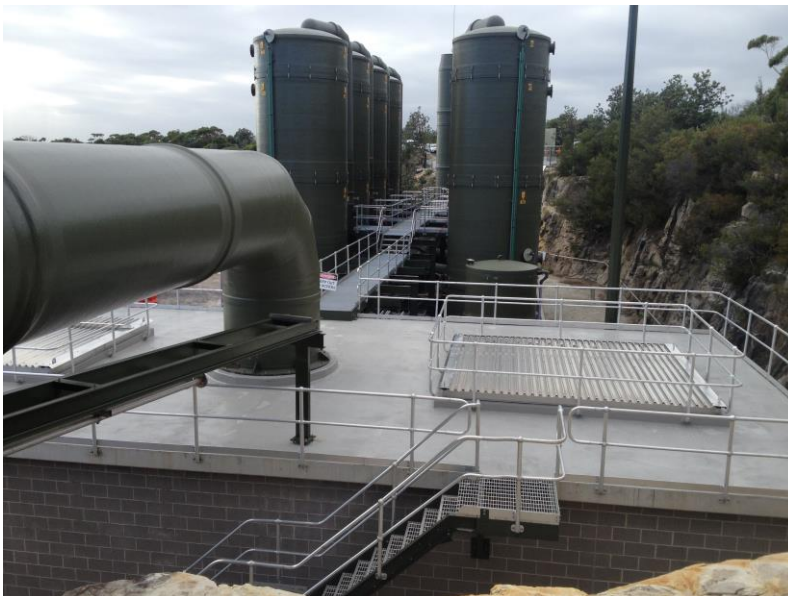
New bio-trickling filters at North Head WWTP
