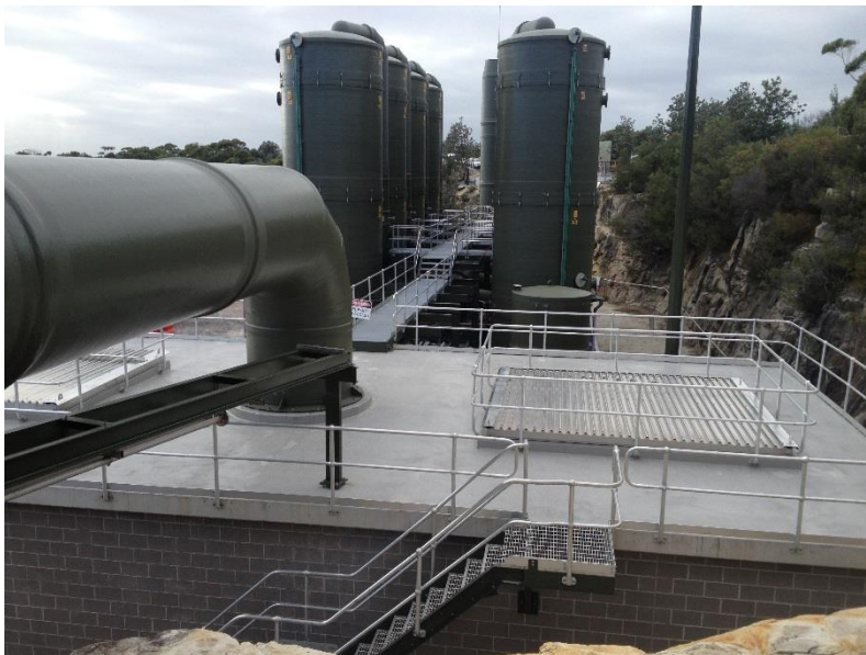
New bio-trickling filters at North Head WWTP
